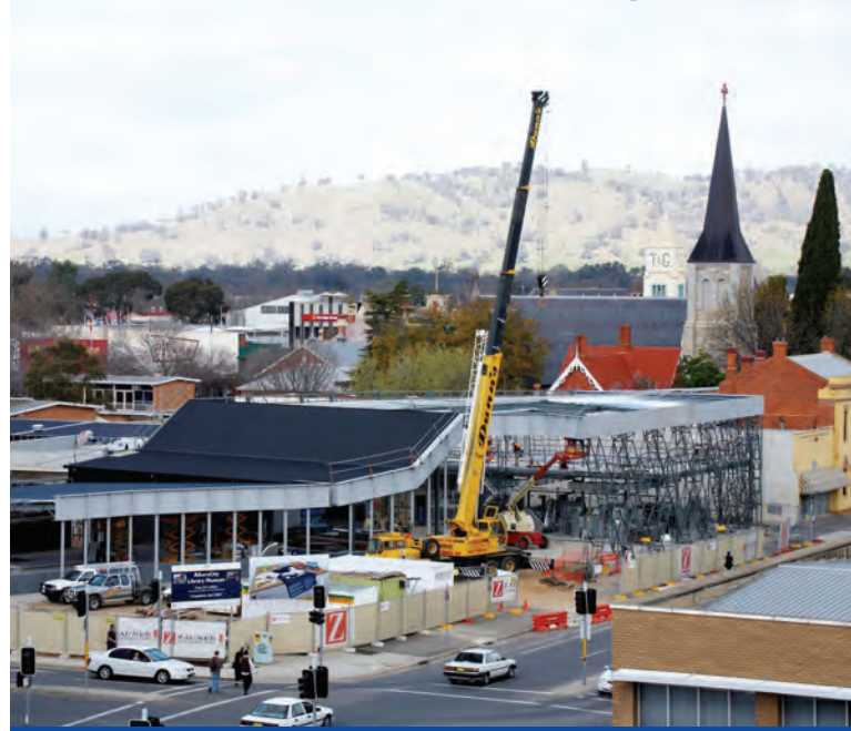
Under construction: Albury City’s new Library Museum, at the forefront of the trend in cultural facilities convergence
